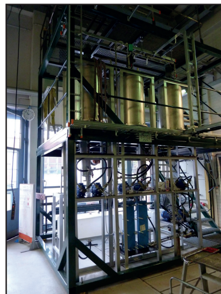
Fig. 5 Photo of the pilot-scale test facility as its current state
